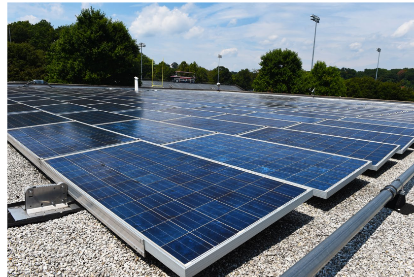
Solar panels on roof of DuFour Athletic Facility
